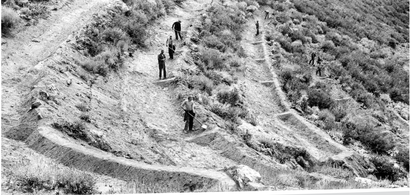
Terrace-trench work, Davis County, c 1935. As one of the New Deal agencies, the Civilian Conservation Corps (CCC) put young men to work building much-needed infrastructure. These terraces and trenches were flood control measures. Image courtesy Utah Historical Society.
